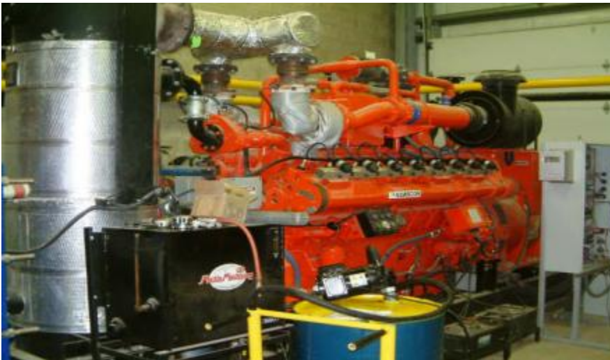
Runs a 720kW genset
