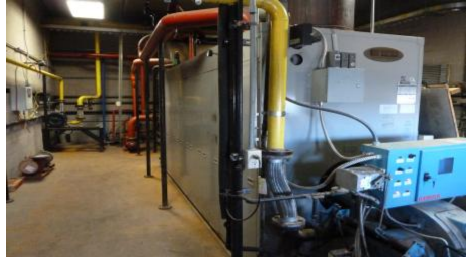
Runs a boiler, which heats the digester
