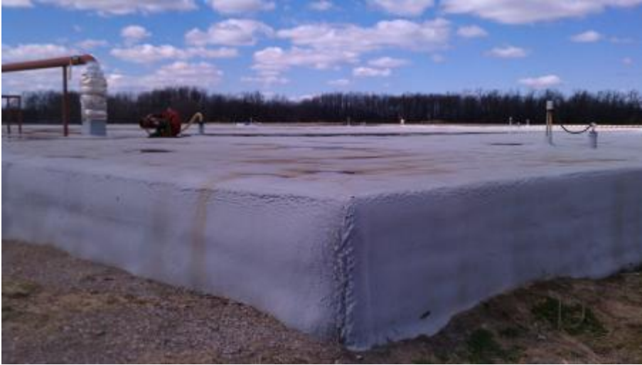
GHD Digester – Mixed Plug Flow, 100F
